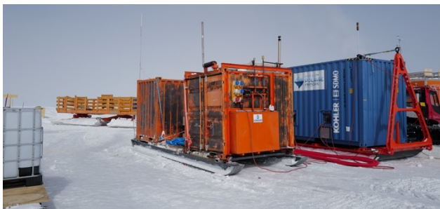
The spare generator. Credit: F. Wilhelms ©PNRA/IPEV
