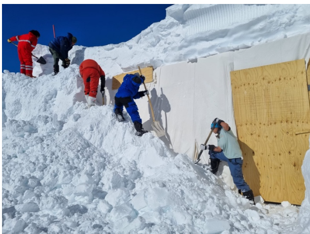
Excavating a ditch to remove load from the trench cover. Credit: L. Ardoin ©PNRA/IPEV
