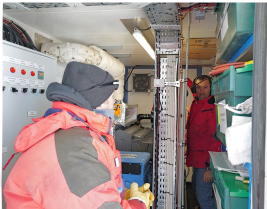
Danilo and Michele switching on the second generator Credit: F. Wilhelms ©PNRA/IPEV
