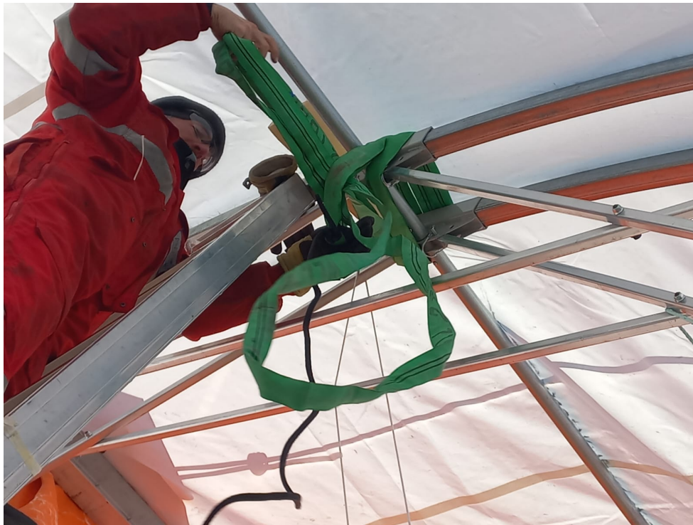
Setting up additional security measures over the drill trench : photo : I. Gay
