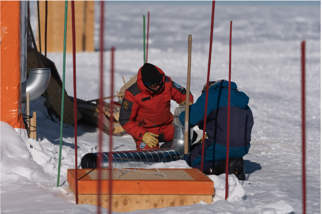
Carlo and Olivier finishing the exhaust pipe for the ventilation. Photo: T. Stocker (Leica SL2-S, 280 mm, f 4, 1/3200 s, ISO-100).
