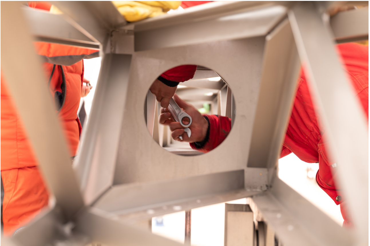
A view through the BEOIC drilling tower during the connection of the tower segments.
