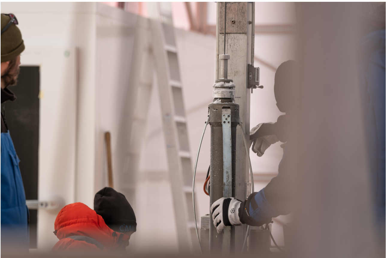
Concentrated work in the BEOIC drilling tent. Romain, Carlo and Philippe are cleaning the hole from reaming debris.
