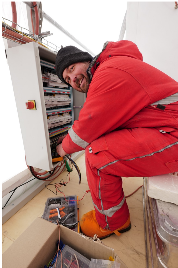
Matthias working on the electrical bard. Photo: T. Stocker (Leica SL2-S, 16 mm, f.1, 1/100, ISO 200)
